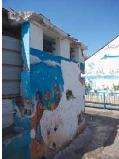
Damage to wall, UNRWA shelter, Jabalia Elementary Girls School, north Gaza. Photo by LBR, 19 Aug 2014
