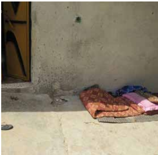
Damage to inner yard of clinic, where Samia Abu Dakka was lying, Khuzaa. Photo by HPH, 10 Sep 2014
